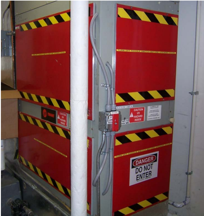
Figure 1. Air handler unit with UV germicidal lamp inside, showing appropriate warning signs.
