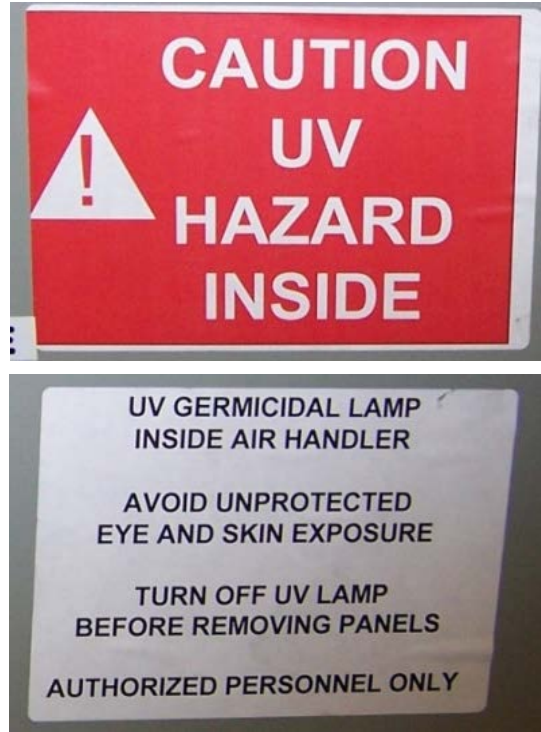
Figures 2-3. Close detail of the warning labels used on the air handler unit in Figure 1.
